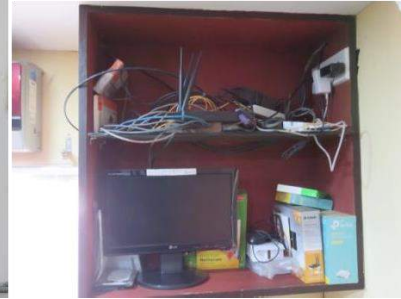
Main Server Computer
