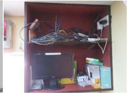
Main Server Computer Entire
