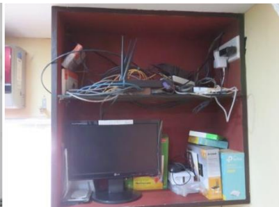
Main Server Computer
