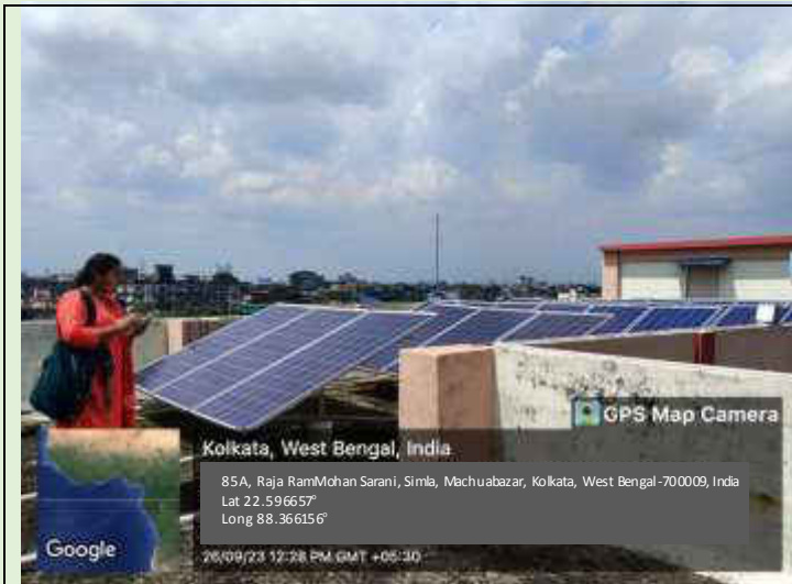
Installed Roof Top Solar Panel
