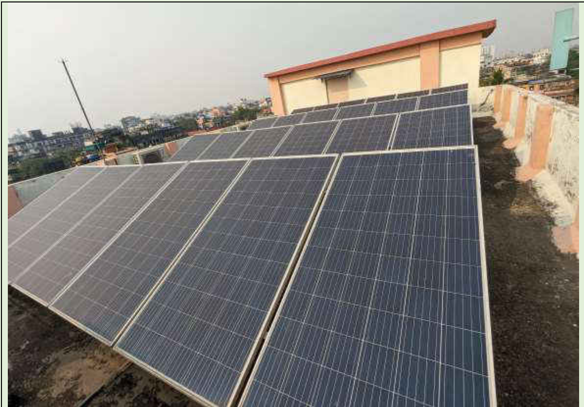
Installed Roof Top Solar Panel
